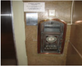
Yule House_fire extinguisher ground floor_KJ_Oct 09
