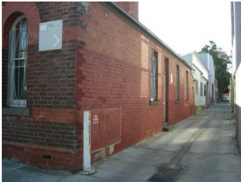
View from Selwyn Street along un-named laneway, showing painted areas of face brickwork on south elevation
