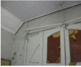
Timber-boarded ceiling junction with south and west walls inside the former fire engine room
