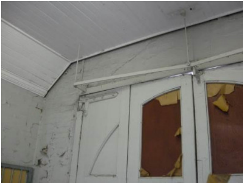
Timber-boarded ceiling junction with south and west walls inside the former fire engine room
