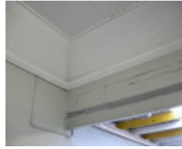
Steel lintel supporting a remnant of the 1896 building's east wall in the north-east corner of the former fire engine room
