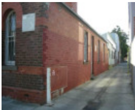
View from Selwyn Street along un-named laneway, showing painted areas of face brickwork on south elevation
