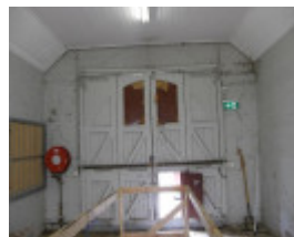
Looking west at the timber and glass doors to the former fire engine room
