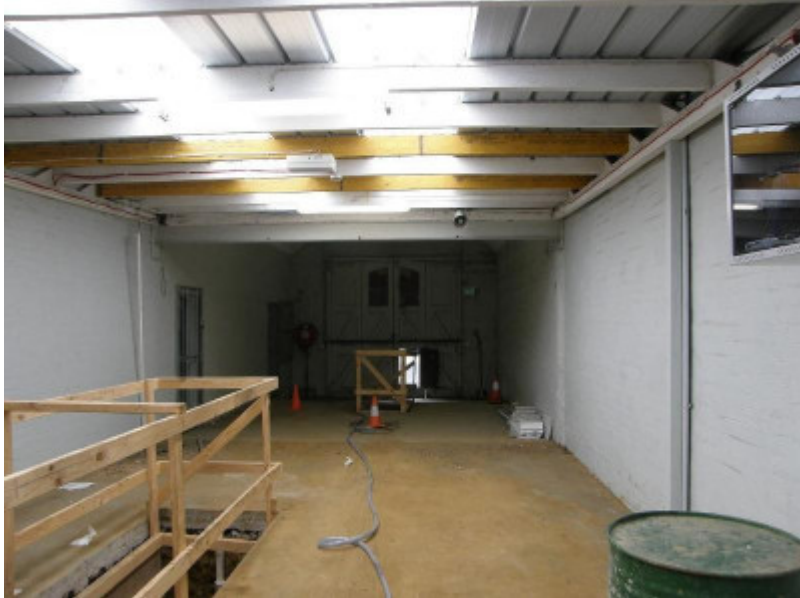
Looking west towards the fire engine room from the space formed by the mid-1950s roofing of the former yard
