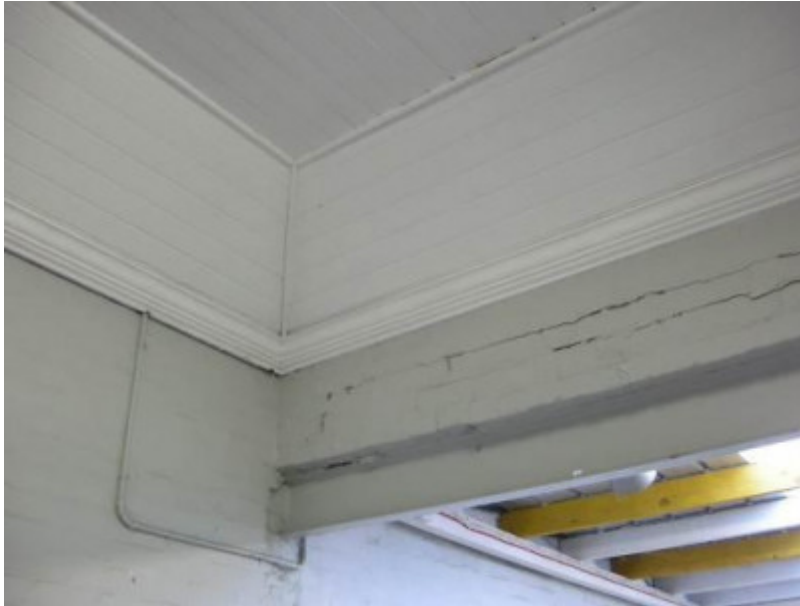
Steel lintel supporting a remnant of the 1896 building's east wall in the north-east corner of the former fire engine room
