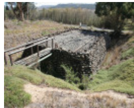
H2167 Lady Northcote Camp Sewerage System
