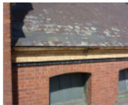
Before Photograph - Reference F3838 2014
