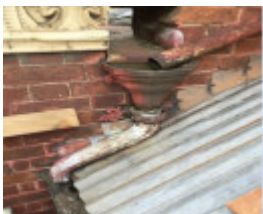
Before Photograph - Reference F3838 2014
