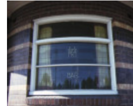
former united kingdom hotel queens parade clifton hill detail of front window
