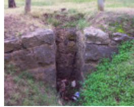
Stonework beside the Toolern Creek. This secured a pipe which supplied water to the reservoir from a small dam on the creek
