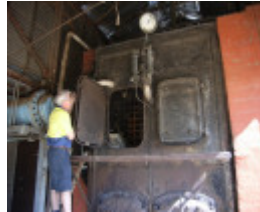
LOCK NINE PUMPING STATION SOHE 2008
