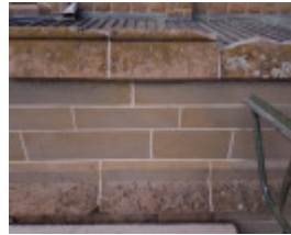
Before Photograph - Reference F3890 2014
