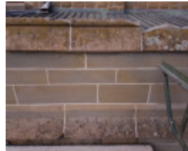
Before Photograph - Reference F3890 2014
