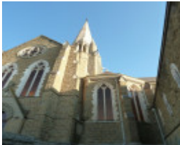
Before Photograph - Reference F3890 2014
