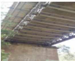
A view from the cycle path at the southern end of the bridge.jpg
