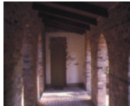
st margaret's church & original vicarage pitt street eltham external entrance arches oct1978
