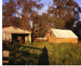
stone cellar at faithfuls creek hume hwy euroa view of property prior to damage
