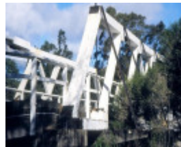
h01214 timber truss and concrete bridge over genoa river genoa northern end she project 2003
