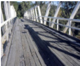
h01214 timber truss and concrete bridge over genoa river genoa decking she project 2003
