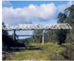
h01214 1 timber truss and concrete bridge over genoa river genoa western side she project 2003
