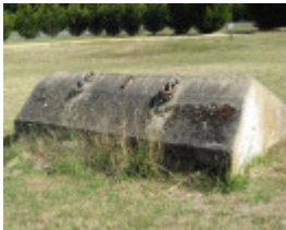
Fiskville concrete block for guy wire anchor
