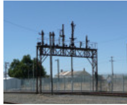
SIGNAL BOX A AND SIGNAL POSTS SOHE 2008
