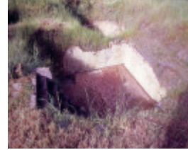
h01330 former thoona dairy and butter factory sargeant street thoona over exit tunnel she project 2004
