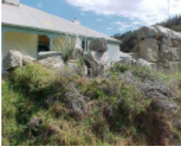
h01983 pt hicks drywall damage2 sep03 pm1
