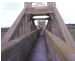
barwon river ovoid sewer aqueduct barwon river geelong view of top aug1988
