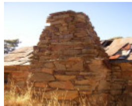
h01743 stone cottages blakeley road barkers creek cottage detached chimney bldg one she project 2004
