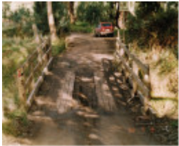
Timber Trestle Bridge Arthurs Creek Eagles Nest Rd Colour 1 - Shire of Eltham Heritage Study 1992
