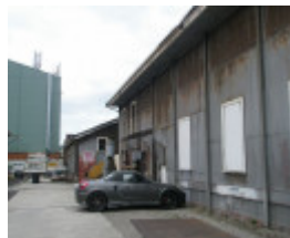
Before Photograph - Reference F3916 2014
