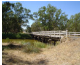
h01850 danns bridge over bet bet creek dunolly eddington road eddington long view she project 2004
