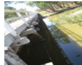
h01850 danns bridge over bet bet creek dunolly eddington road eddington railings she project 2004
