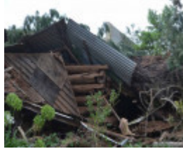
B3239 Storm Damage March 2012
