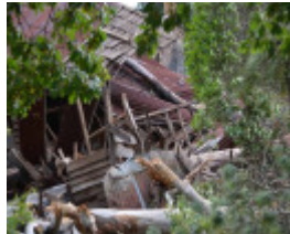
B3239 Storm Damage March 2012
