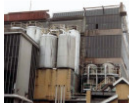
B5089 Main Refinery & New Boiler
