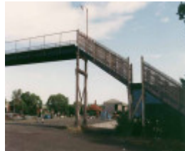
B7125 Nth Fitzroy Railway Footbridge
