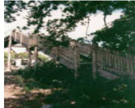
B7125 Nth Fitzroy Railway Footbridge
