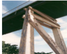
B7125 Nth Fitzroy Railway Footbridge
