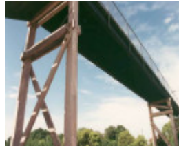
B7125 Nth Fitzroy Railway Footbridge
