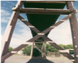
B7125 Nth Fitzroy Railway Footbridge
