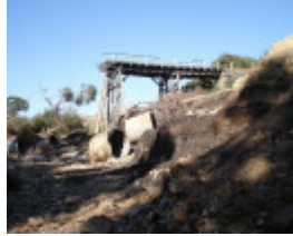
B6923 Springdallah Bridge remnants
