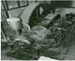
B6329 Rokeby Pumping Station
