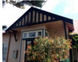
'Flying' gable, 14 Bridge St
