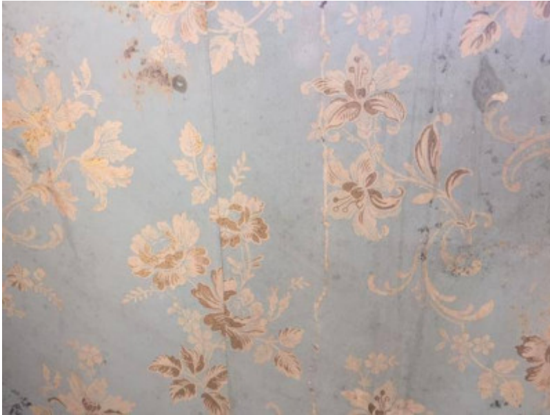
Photo_1.JPG Sample of remnant original wall finish to Room1.138 (south west wing) dating to 1880-81.
