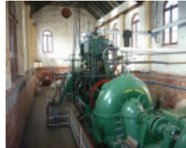
PSYCHE BEND PUMPING STATION SOHE 2008
