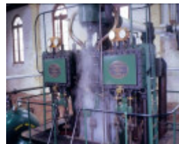
h00548 psyche bend pumping station psyche bend mildura engine room close up she project 2003
