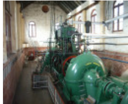
PSYCHE BEND PUMPING STATION SOHE 2008
