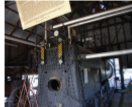
PSYCHE BEND PUMPING STATION SOHE 2008
