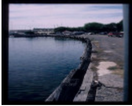
WILLIAMSTOWN SEA WALL & DRAIN
