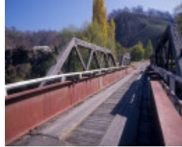
h00917 hinnomunjie bridge over mitta mitta river omeo from omeo end she project 2003
