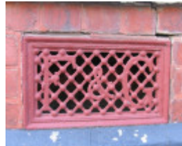
Distinctive 'F & G' air vent
