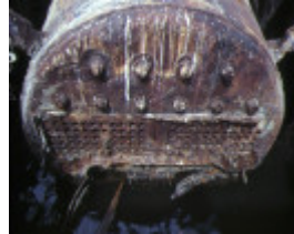
S333 HenryMeakin PortPhillipBayCorioBay Boiler
